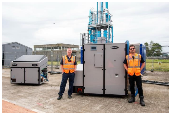
Figure 3. Image of the HERU unit at R2IC (Spernal WWTW)
